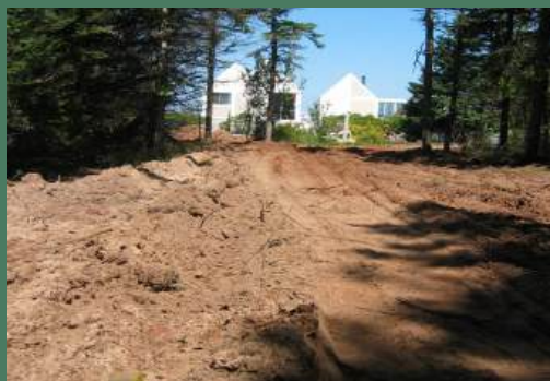
Effluent force main from cottages to septic field.
