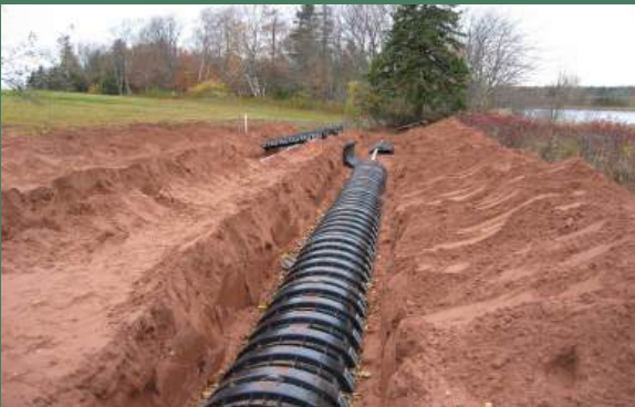
Leaching chambers adjacent to wetlands.
