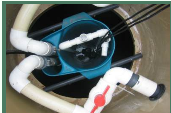
Duplex pumping system inside the OSI screened vault.
